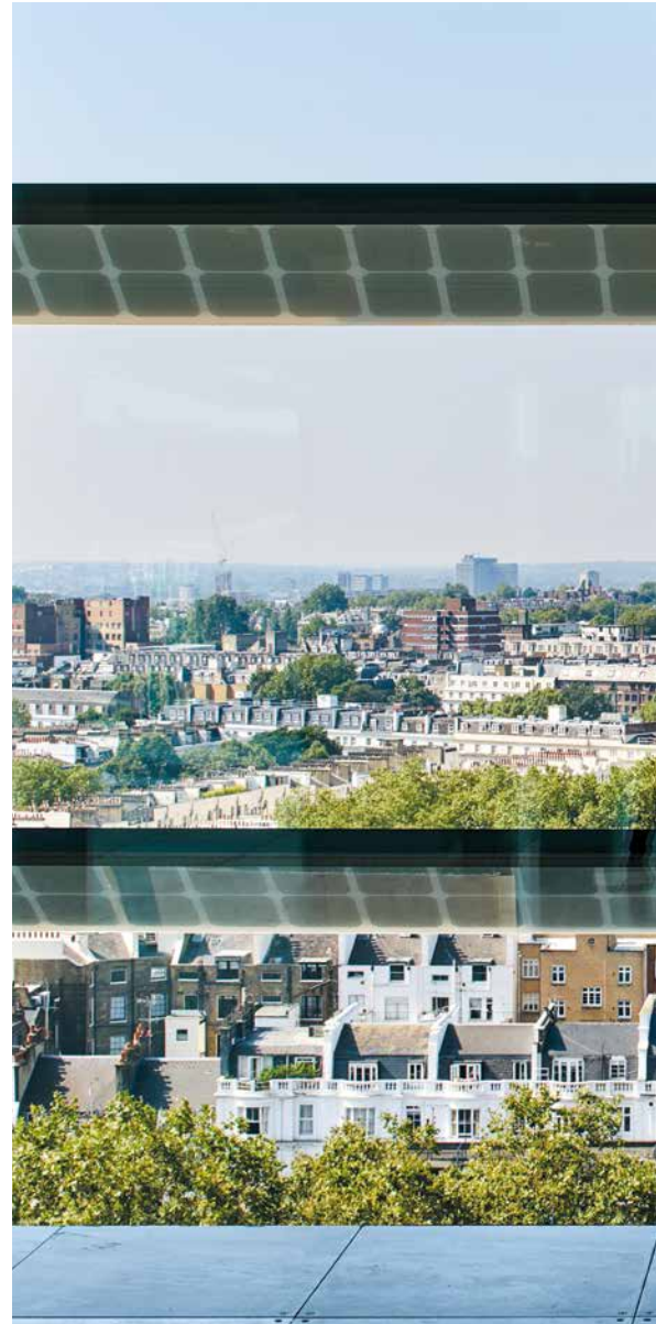
Solar louvres at 20 Eastbourne Terrace, W2
